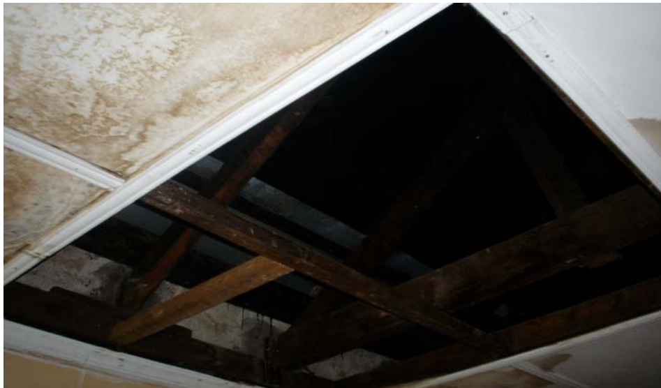
A present image of the roof alleged to have been repaired three times
